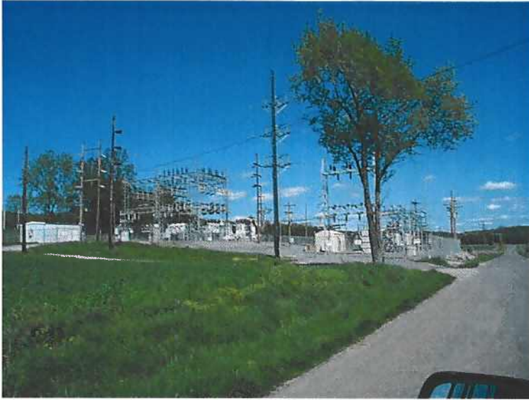
Large electric substation
